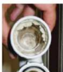
Same pipework—using Biological Urinal Blocks
